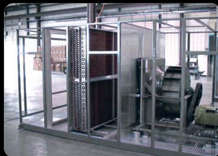
Conventional air-handler fan section
