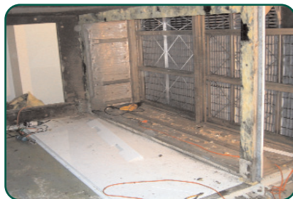
FANWALL array took less space, lowered sound levels, and reduced required motor power by 50%—from 39 FLA to 21 FLA
